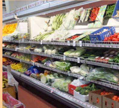
Open fridges like this can be retrofitted with doors that reduce energy use. 16
