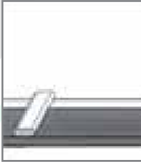
Cable running across plaster board ceiling
