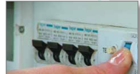
Fuse and circuit breaker
