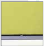
Cable running across the top of a plasterboard ceiling which is covered with thermal insulation
