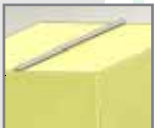
Cable running across the top of insulation
